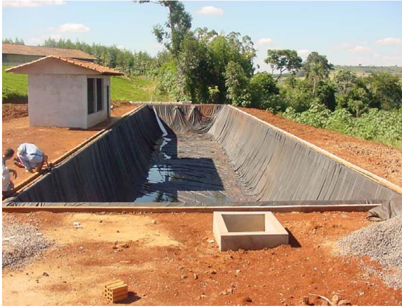
Fig. 2 – Anaerobic digester implantation at Luz Marina – Granja 8 – Toledo – PR
